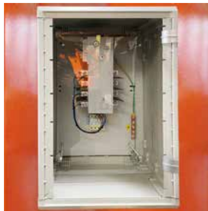
QTC OUT - located outside the generator
