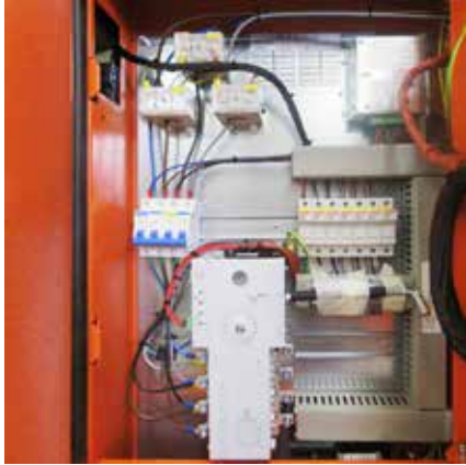
ATS IN - located inside the generator's electrical panel
