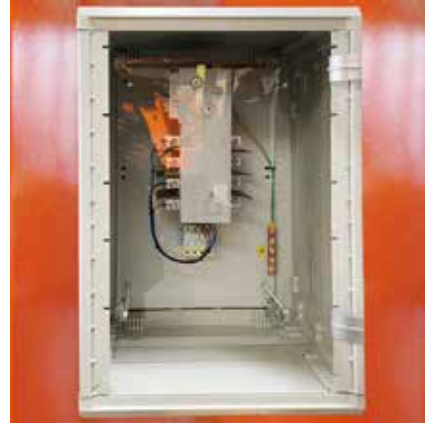
ATS OUT - located outside the generator
